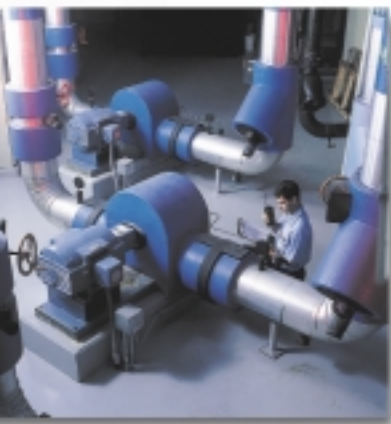
Traditional pump room application for VFD's
